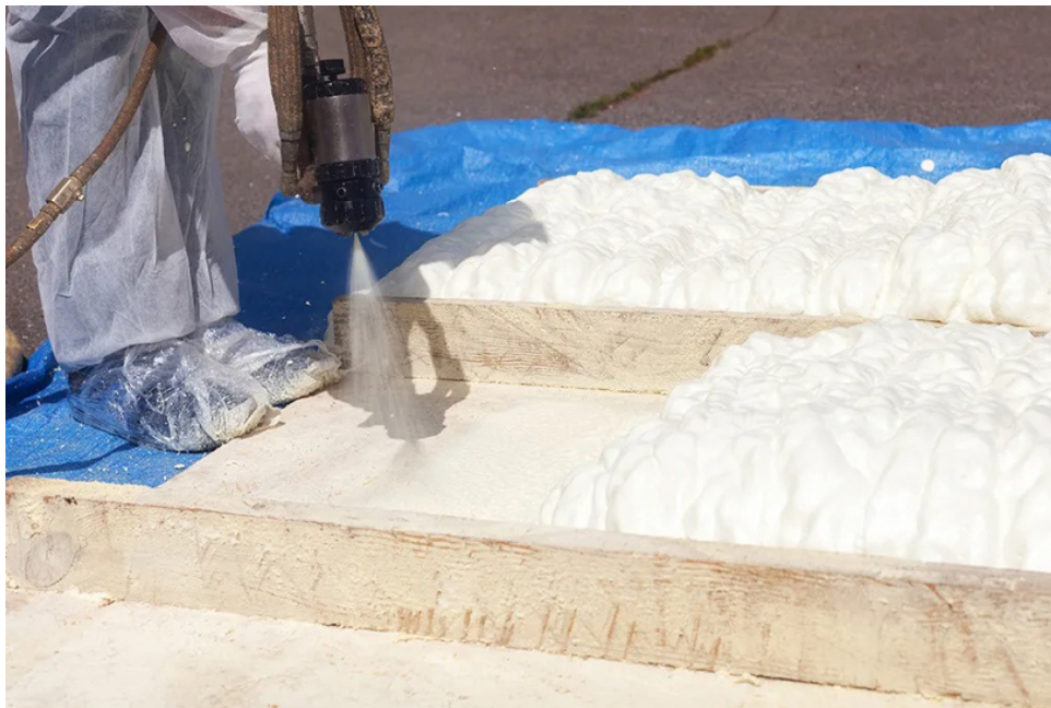
Polyurethane roof insulation
